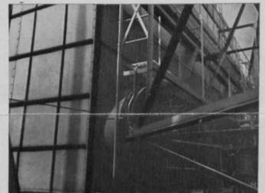
Steel Cooling Tower Protected with Bitumastic No. 50.
